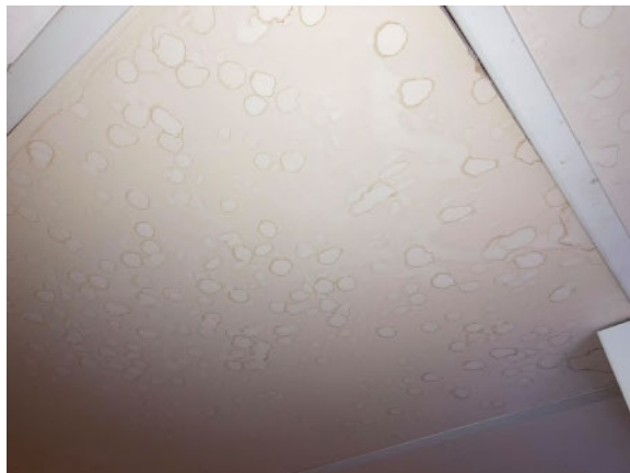
Representative photograph of a ceiling panel within the female bathroom, at the time of the inspection
