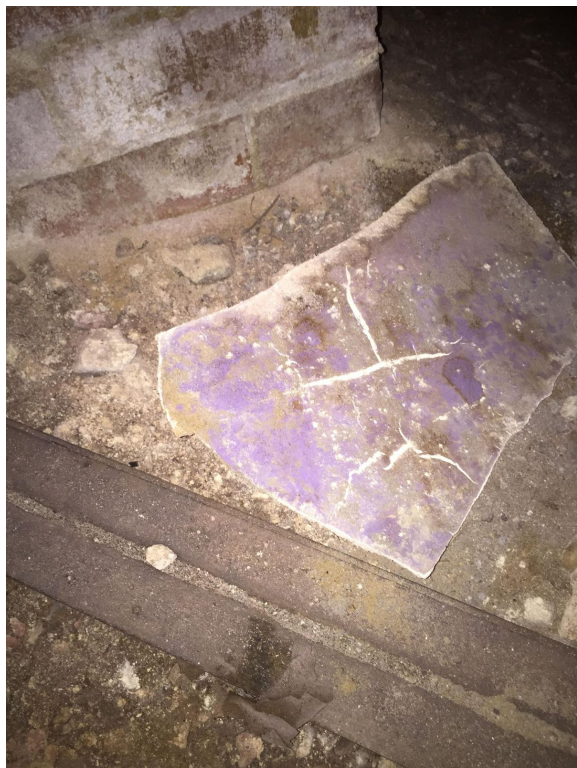
Representative photograph of remnant fibrous cement sheeting within the subfloor
