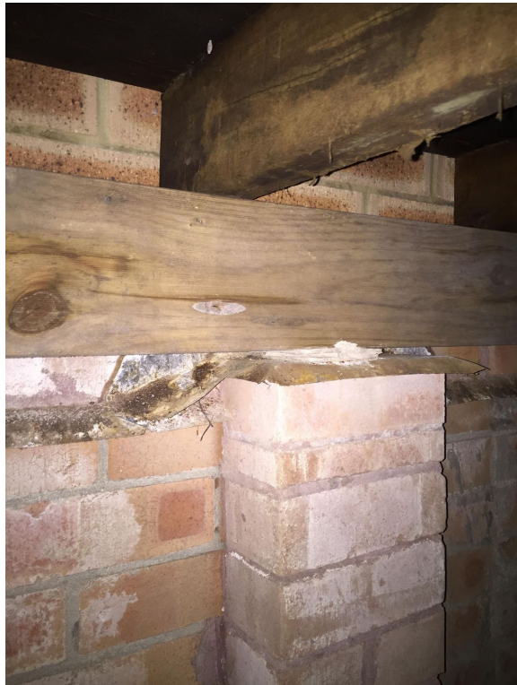
Representative photograph of fibrous cement packers supporting the timber bearers
