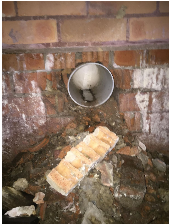
Representative photograph of one of the pipes along the western wall of the subfloor
