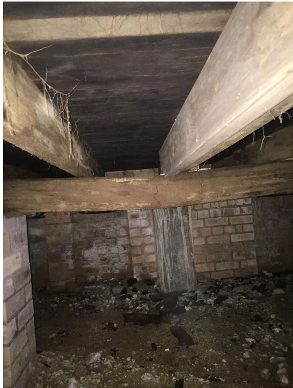
Representative photograph of a fractured floor timber bearer
