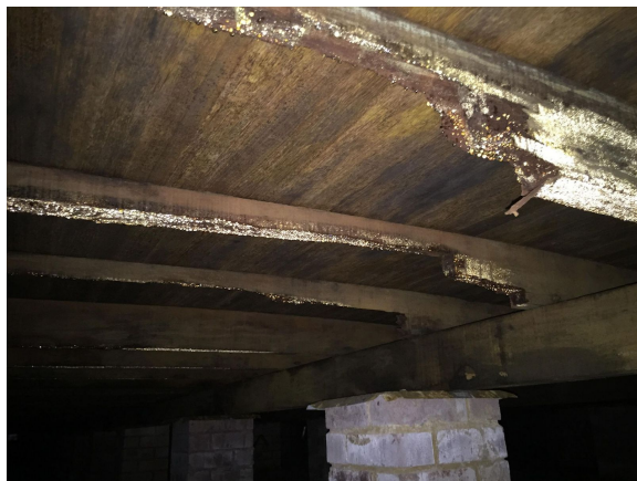
Representative photograph of several floor timber joists that have partially broken and are coated with moisture
