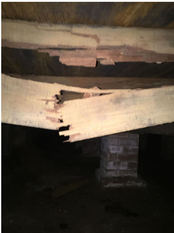
Representative photograph of a broken floor timber joist within the subfloor
