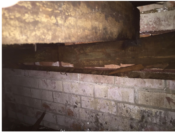
Representative photograph of a floor timber bearer immediately adjacent the northern brick wall
