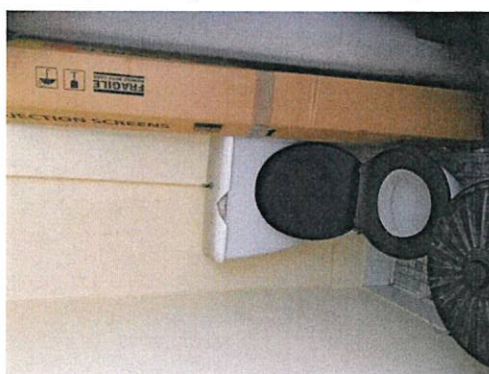
Sanitary Plumbing - Toilet - China Bowl/Cistern
