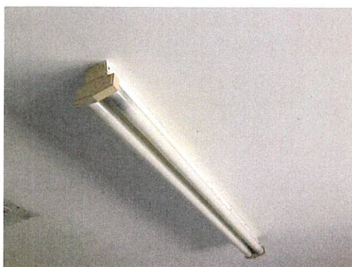
Lighting - Fluorescent Lights
