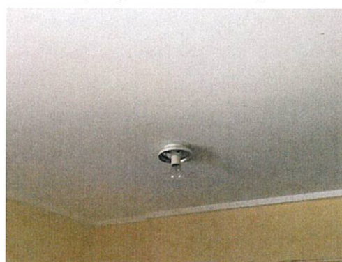
Lighting - Incandescent Lights
