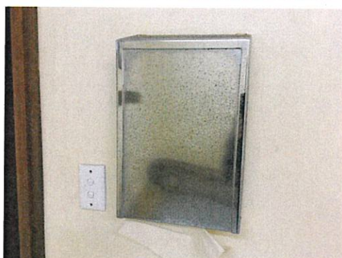
Fixtures & Fittings - Paper Towel Dispenser
