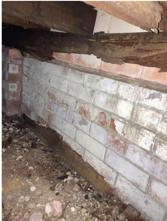
Representative photograph of the northern brick wall covered with a white powdery substance, at the time of the inspection
